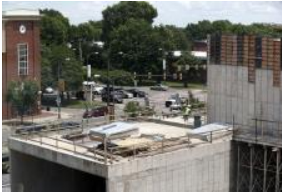
The VCU Institute for Contemporary Art is being constructed at the corner of West Broad and North Belvidere Streets Wednesday, June 29, 2016.
